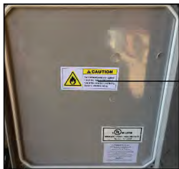
INSIDE OF ELECTRICAL BOX
